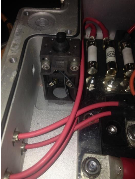
Switch in HVJB
