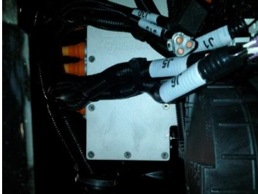
High Voltage Junction Box (HVJB)
