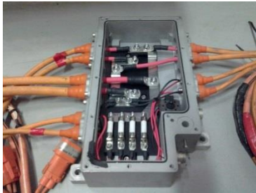
HVJB – Cover Removed
